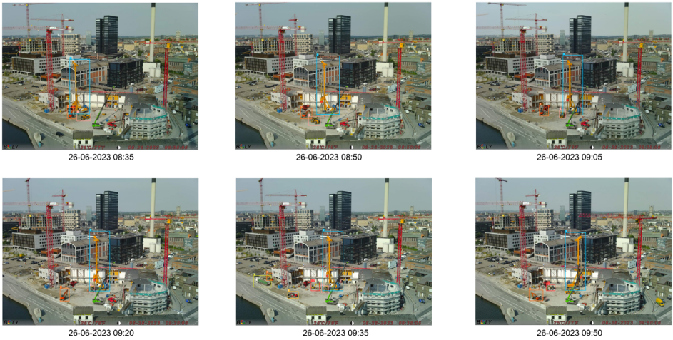
Figure 6. Detection of equipment and its operation status on 26-06-2023
